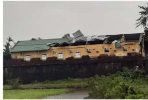
Figure 2: First Damage of Vamco in Military hospital in Hue city
